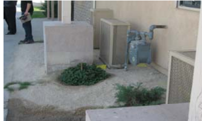
Sidewalk Utility Boxes
