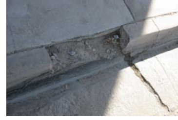
Deteriorating Curb Face
