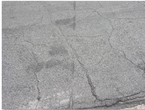
Example of Alligator Cracking
