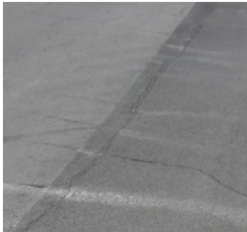
Example of Longitudinal Cracking
